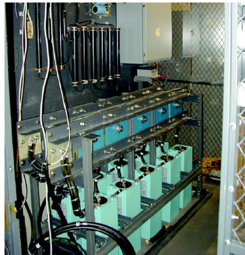
Figure 2.2.3.3.3-4: The NSTX CHI capacitor bank system is well suited to powering the EPI injector for NSTX-U.
