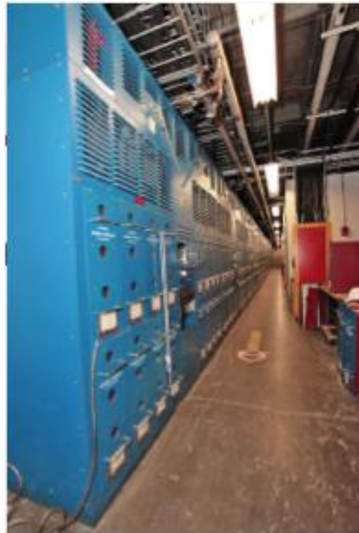
Fig. 10.20. Photograph of the FCPC facility.
