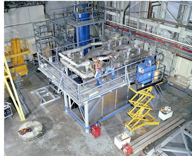
Lid stand holding BL lid with cryo manifolds and panels (photo circa 1980)
