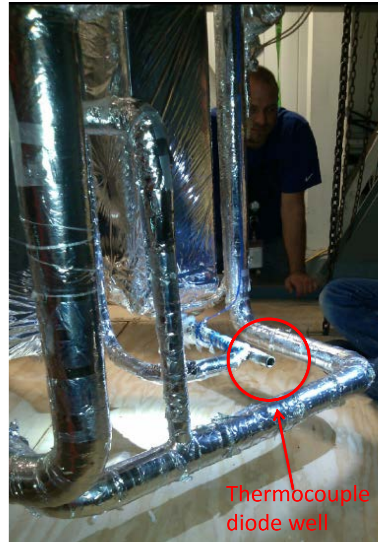
Interior of the LHe Refrigerator Cold Box
