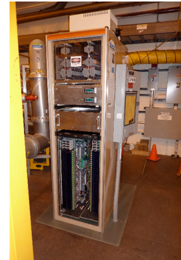
Control Rack Installed
