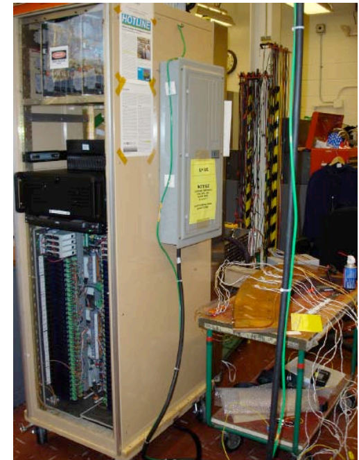
LLD Control Being Tested Off-Line
