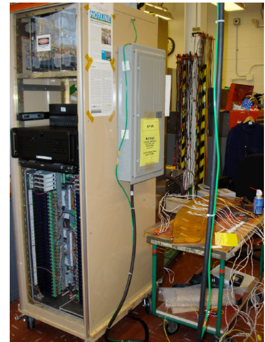
LLD-1 Control Being Tested Off-Line
