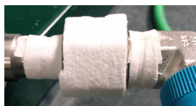
The copper shell is stood off from the pipe by insulating ceramic tape.
