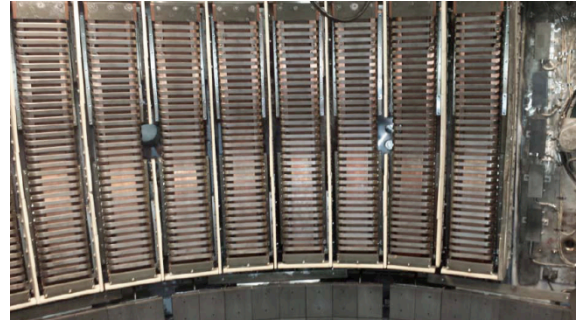
FIG. 5. Enhanced HHFW antenna installed in NSTX-U with compliant feeds and improved back-plate grounding.
