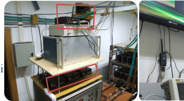
(left) 4 wireless modules installed in the power supply and the timer; (right) The wireless modem attached on the remote computer.
