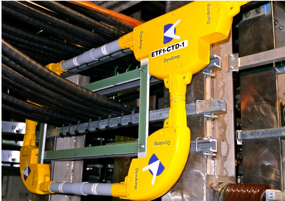
+150/-150kA DCCT installed in TF Circuit
