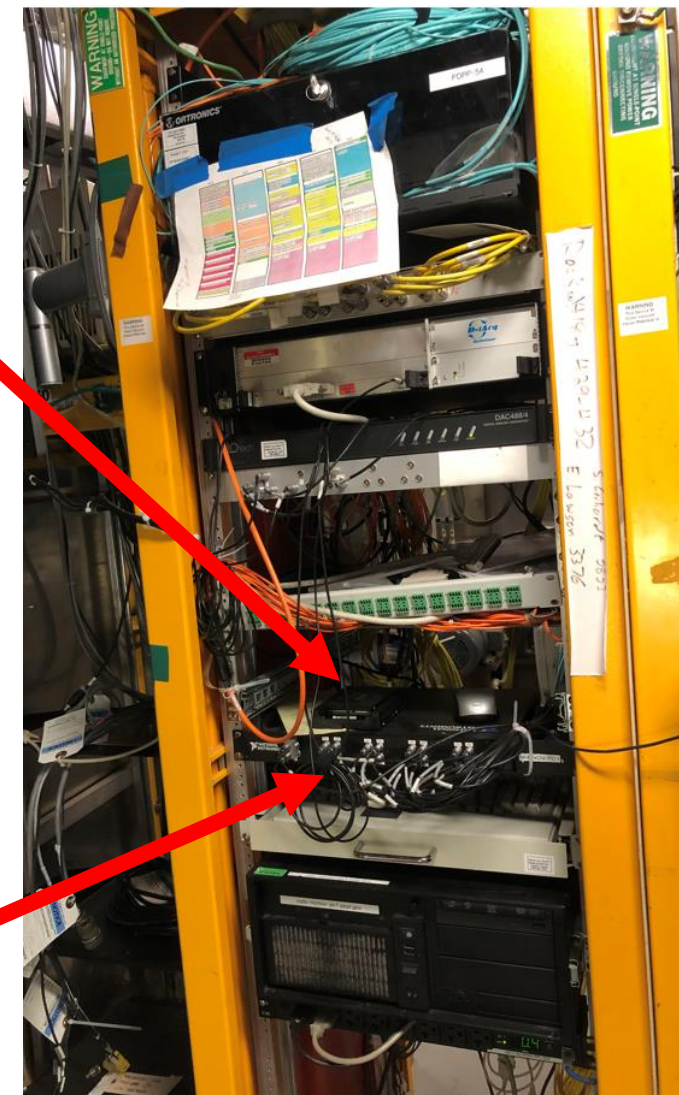
LEMO cables from high-n array mag probes
