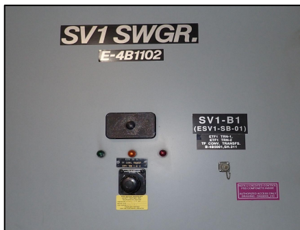
PSS-SIS INSTRUMENTED MEDIUM VOLTAGE BREAKER
