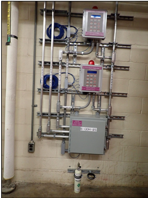
Typical Redundant Monitor Installation
