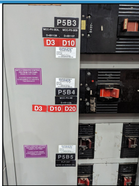
BREAKERS ON THE AC DISTRIBUTION
