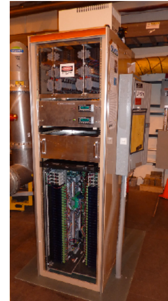
LLD-1 Control Rack in NSTX Test Cell
