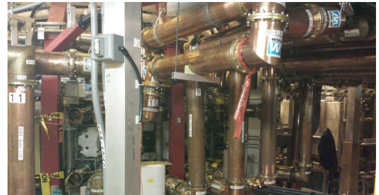
Resonant loop connections to top/bottom antenna element feeds
