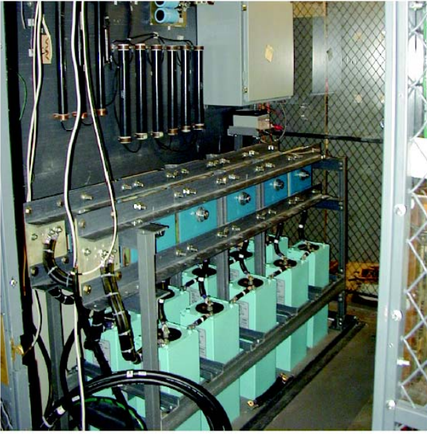
Fig. 4. NSTX-U transient CHI capacitor bank showing the 10 individual capacitors.
