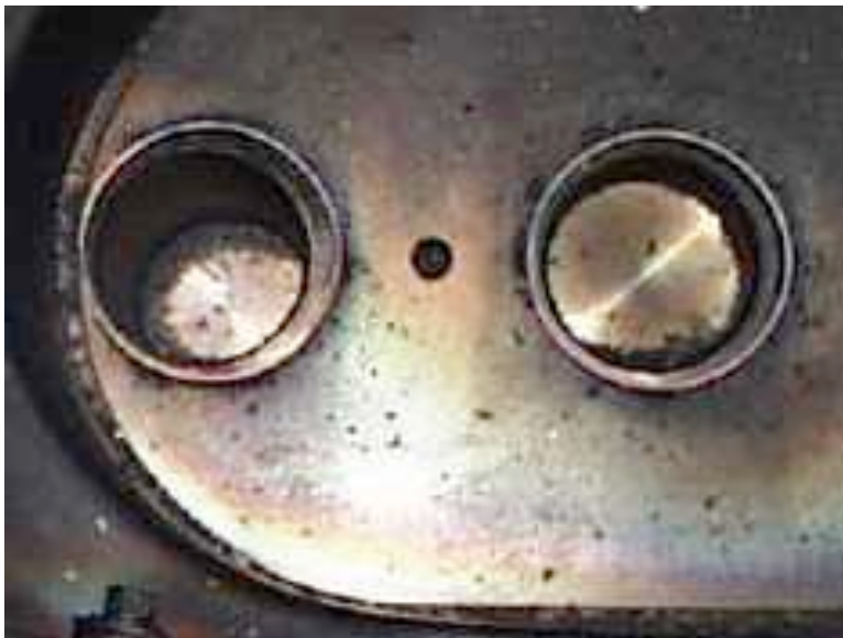
Debris and dust on TFTR vessel floor
