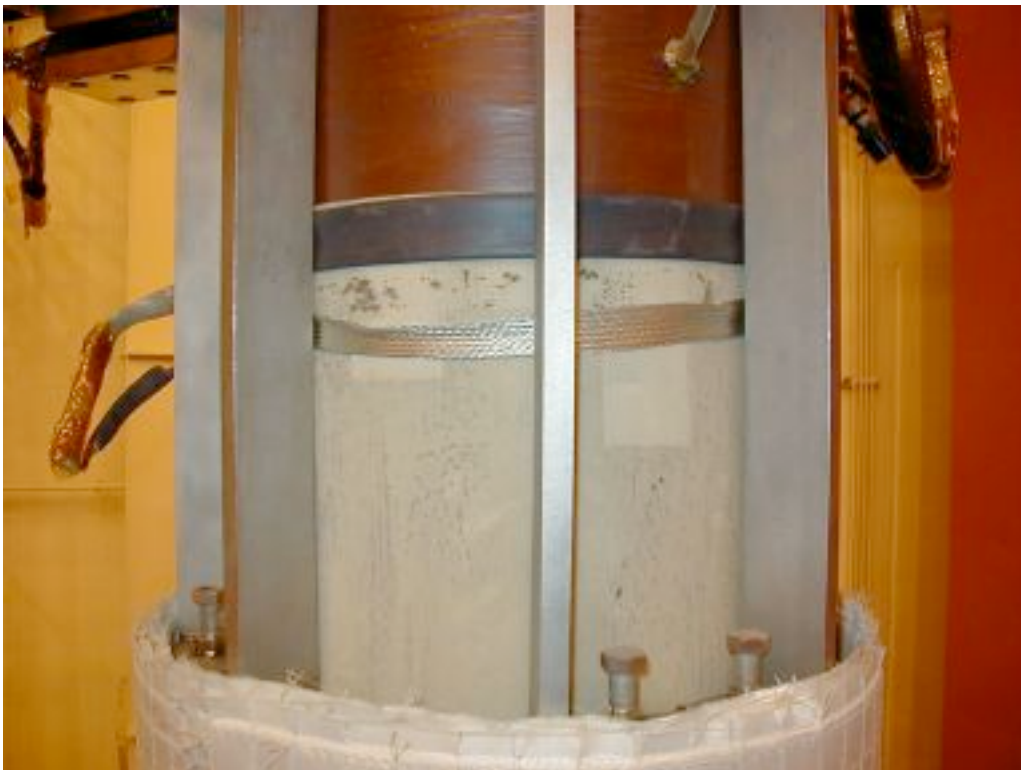
Figure 1 – Pitting Under Existing OH Ground Plane Connector
